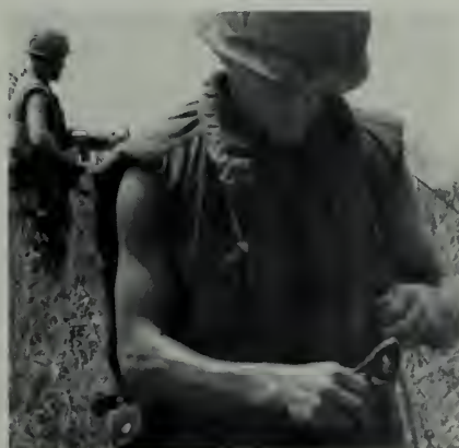
When wire trouble develops, men go into the DMZ to repair breaks.
